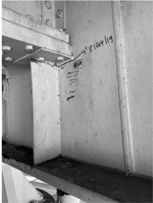
TYPICAL CS CRACK
