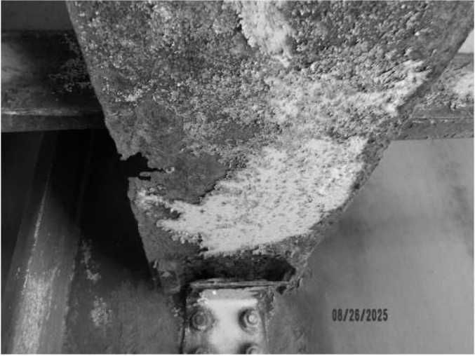
SECTION LOSS – GIRDER B BOTTOM FLANGE
